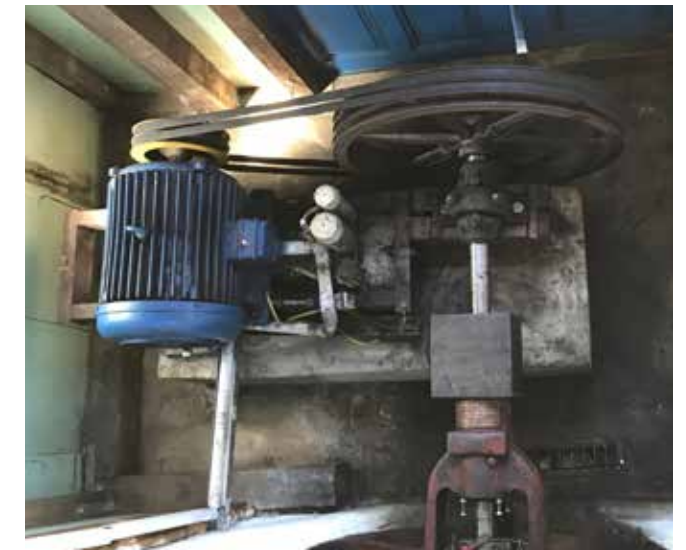
No. 3 Turbine before refurbishment efforts began
